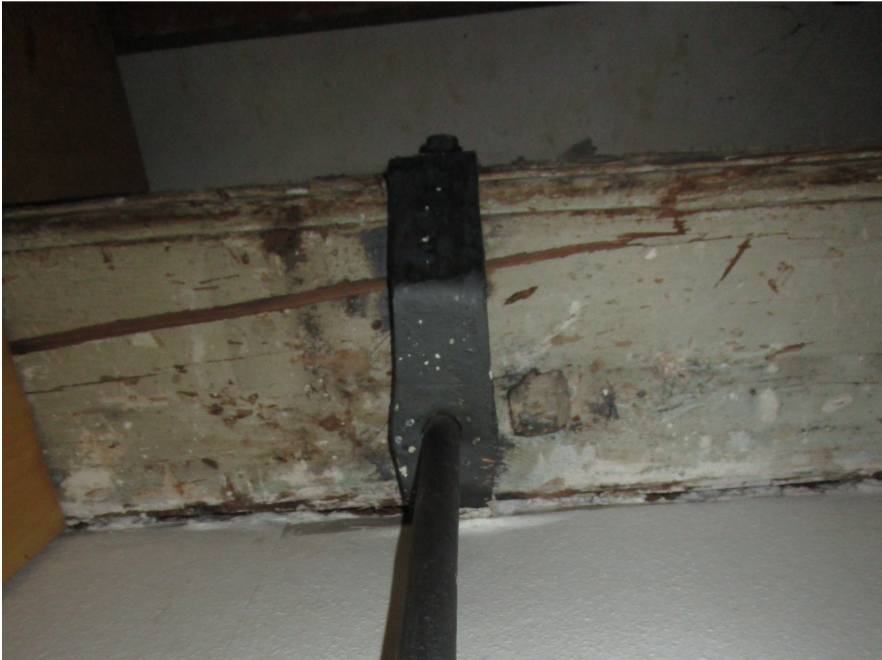
Broken horizontal beam in the pastors' apartment
